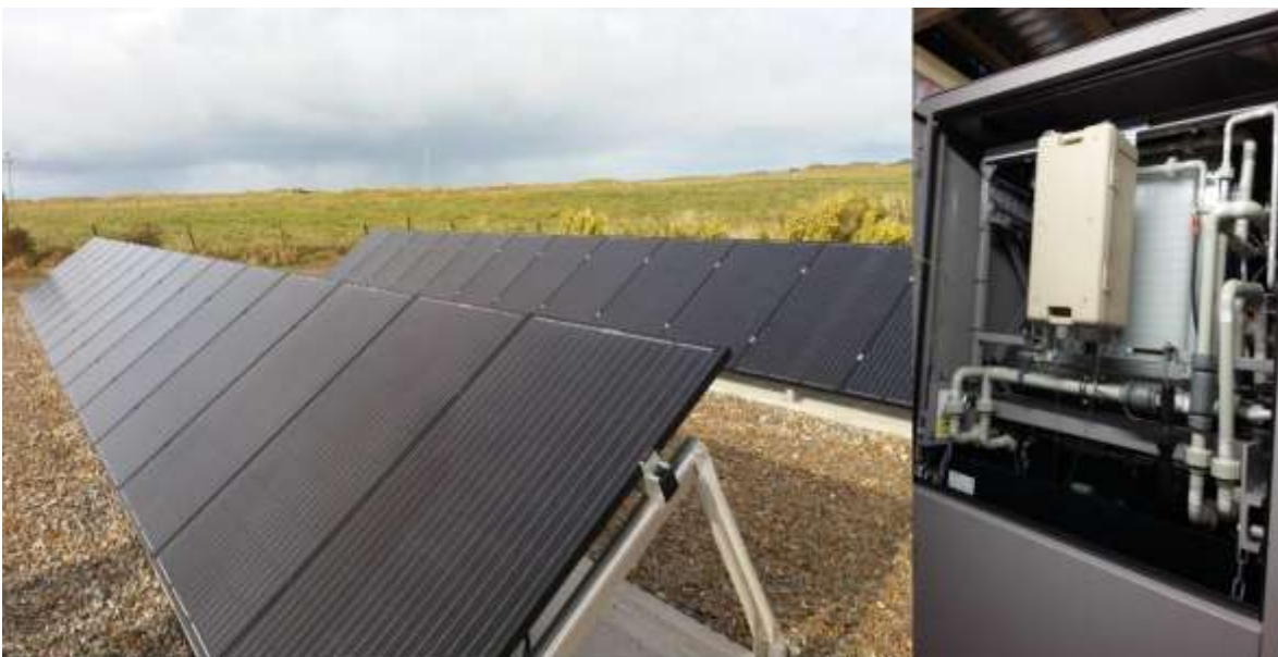
Figure 1. The 11 kW Solar PV and 40 kWh Vanadium battery system at the Each Leim site. 1
