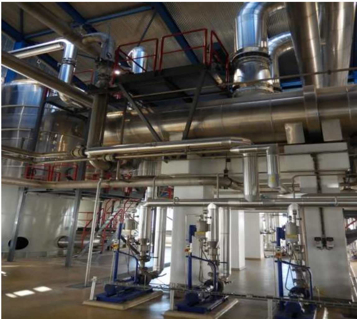
Figure 1. At Svartsengi Geothermal Power Plant. 1
