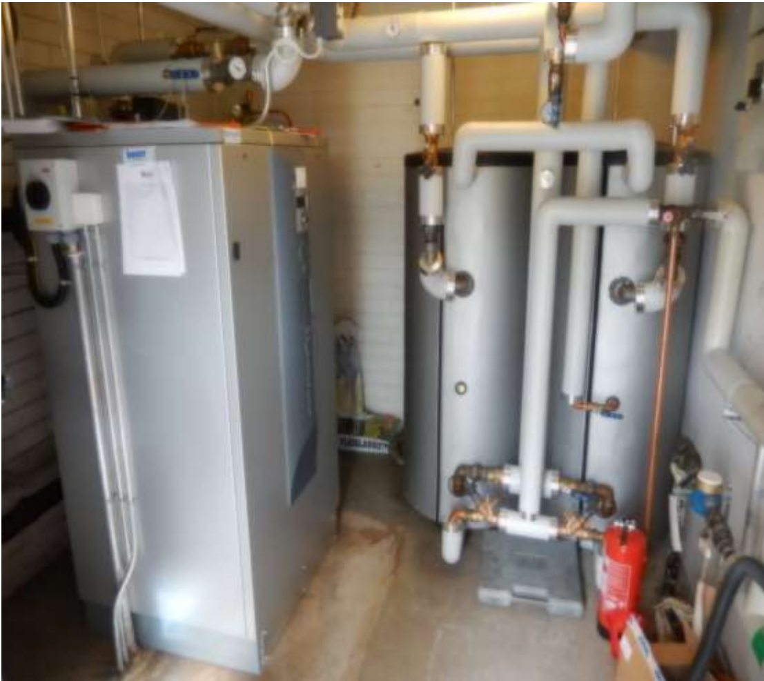
Figure 1. Ground source geothermal.
